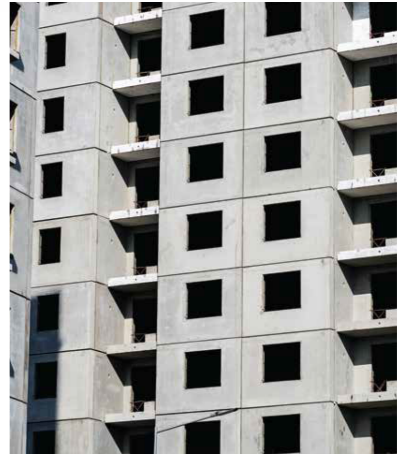
Use of Damp Proof course & Shower test is carried on the external walls to observe any seepages.
